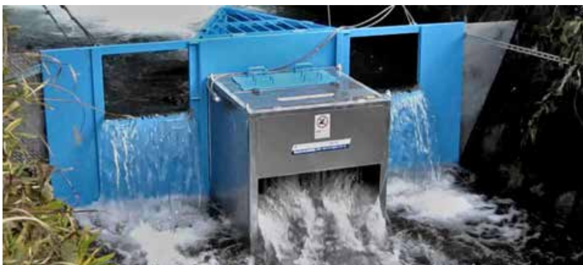
DOMESTIC SMALL HYDRO POWER UNIT INSTALLATION (SOURCE: GOOGLE)
