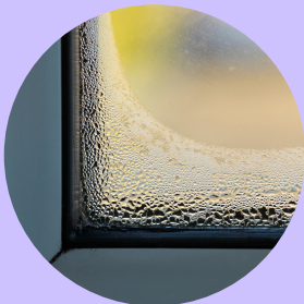
Condensation on an external window
