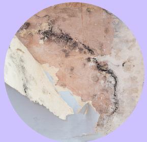
Black mould growing on plasterwork
