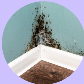
Black mould growing in the corner of a room
