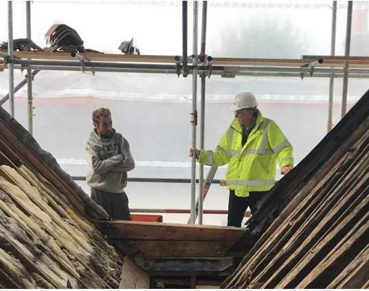
Project manager Steve Collins on the left and architect Simon Plater on the right during re-roofing.
