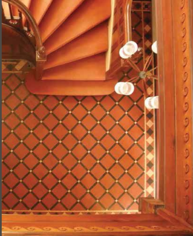
An entrance hall with encaustic tiled floor and grand open-well staircase in a Grade II listed building, c.1880
