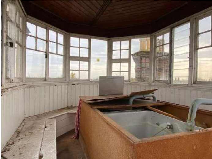
Inside the Belvedere at Mountview prior to restoration. The space was dominated by a large water tank. Several of the original windows had been replaced by unsympathetic louvred windows.
