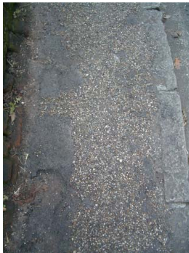
Fig. 17 Bonded shingle pavement surface, in poor condition
