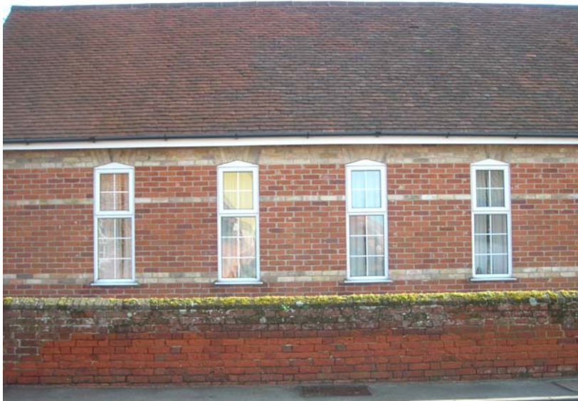
Fig. 64 Plastic replacement windows, old school, Church Street.
