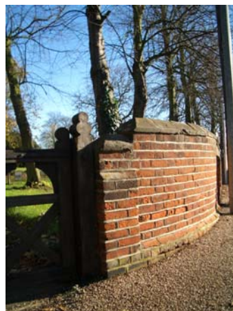
Fig. 12, Red brick wall in Flemish bond (with unfortunate cement repointing)
