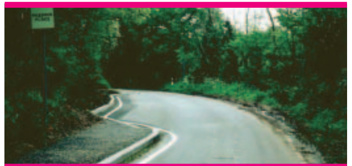
Verge erosion has continued opposite the passing places
